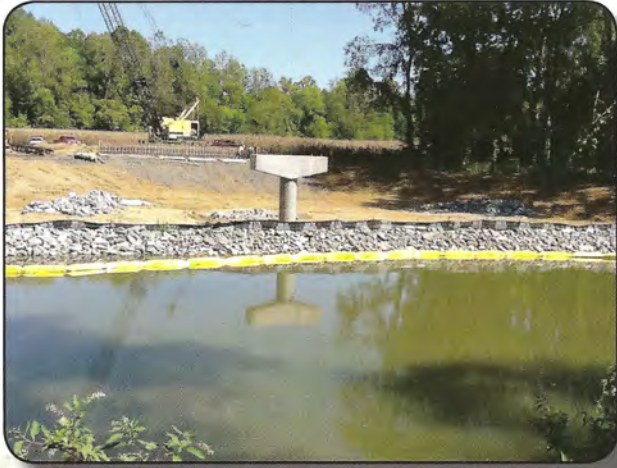
Before: Unsuccessful Rock Rip-Rap
